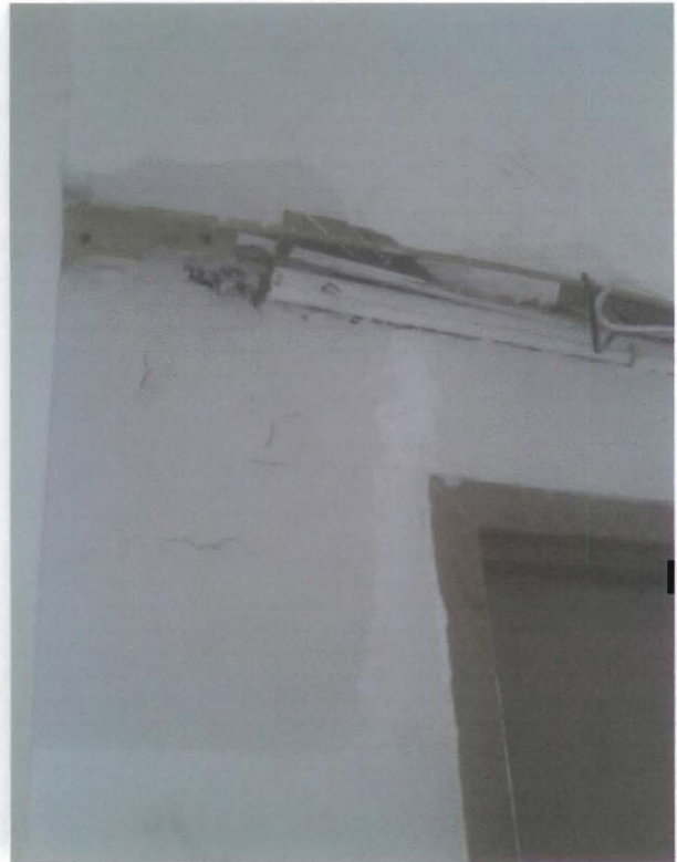
Photo 13 of 13 inadequacies 019.jpg Date: 05.10.2011 12th floor hallway - poorly finished wall "prep" and paint
