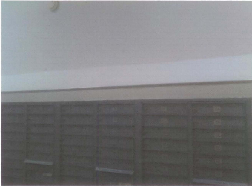
Photo 11 of 13 inadequacies 041.jpg Date: 05.10.2011 Mail room - finish
