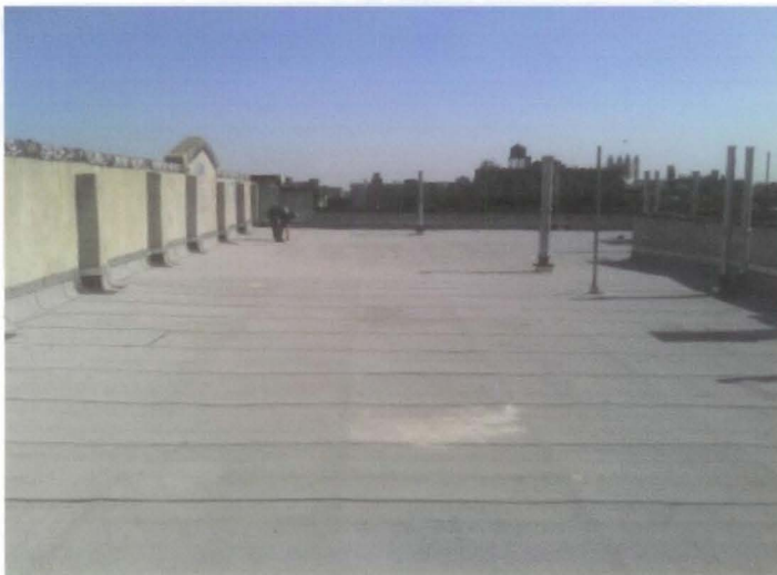
Photo 7 of 13 inadequacies 025.jpg Date: 05.10.2011 Roof
