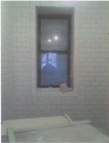
Photo 1 of 3 – Performance Level – 5F bathroom
