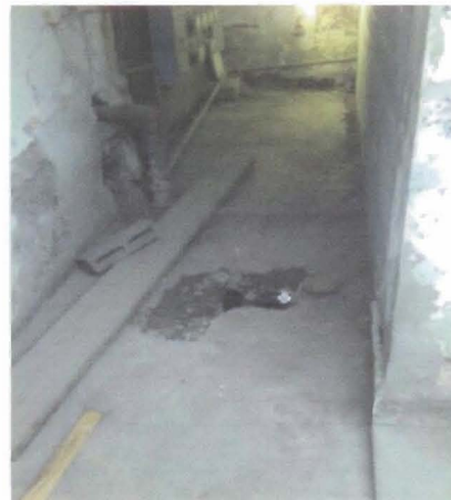
Photo 4 of 4 – Performance Level – basement drain
