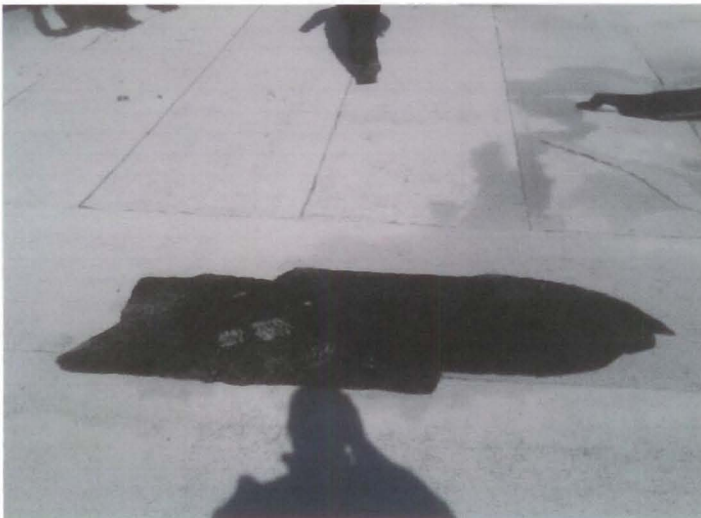
Photo 6 of 13 inadequacies 024.jpg Date: 05.10.2011 Roof - damage to external membrane
