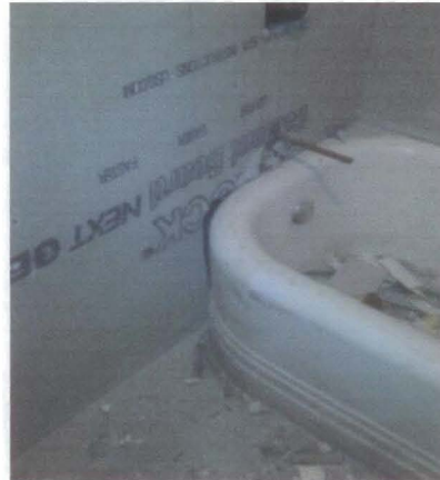
Photo 2 of 4 - Performance level – 1F bathroom
