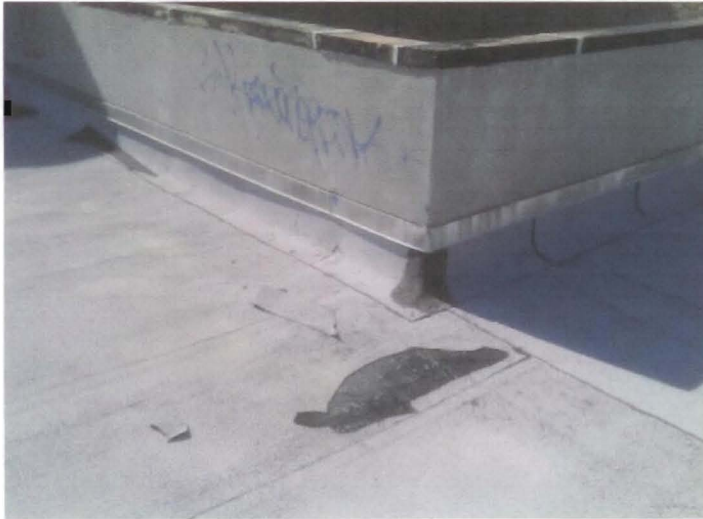
Photo 8 of 13 inadequacies 029.jpg Date: 05.10.2011 Roof - damage to external membrane near parapet wall
