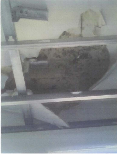
Photo 1 of 13 inadequacies 008.jpg Date: 05.10.2011 12F ceiling water damage liv. Rm.
