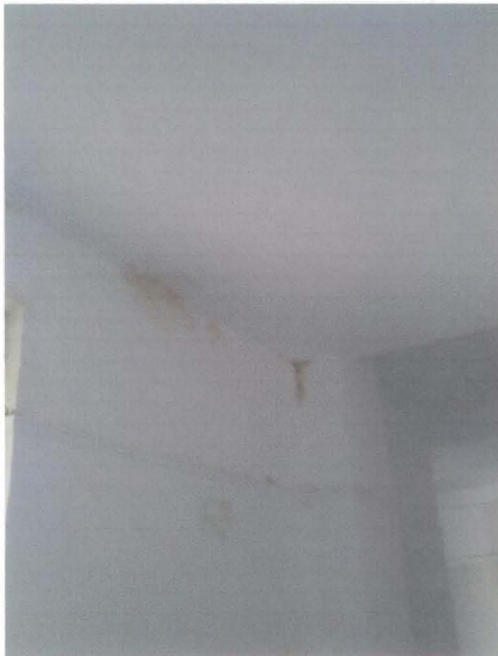
Photo 3 of 13 inadequacies 014.jpg Date: 05.10.2011 12th floor hallway water damage
