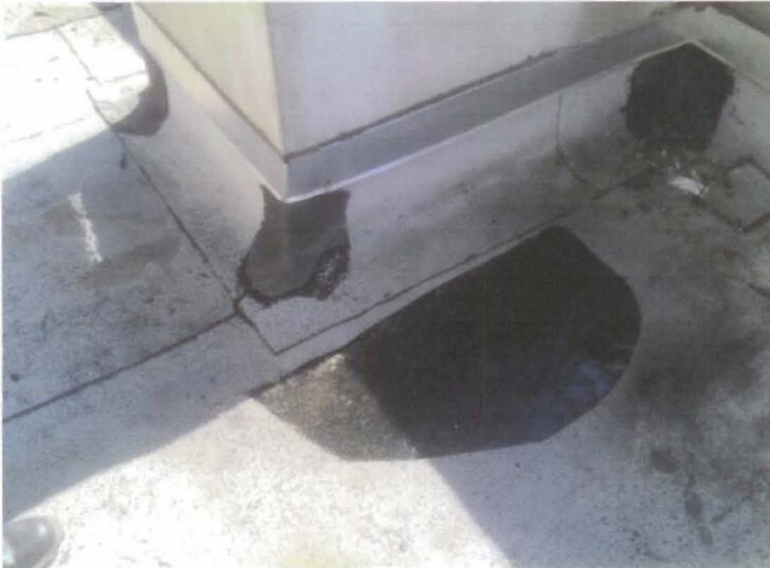
Photo 5 of 13 inadequacies 021.jpg Date: 05.10.2011 Roof - damage to external membrane
