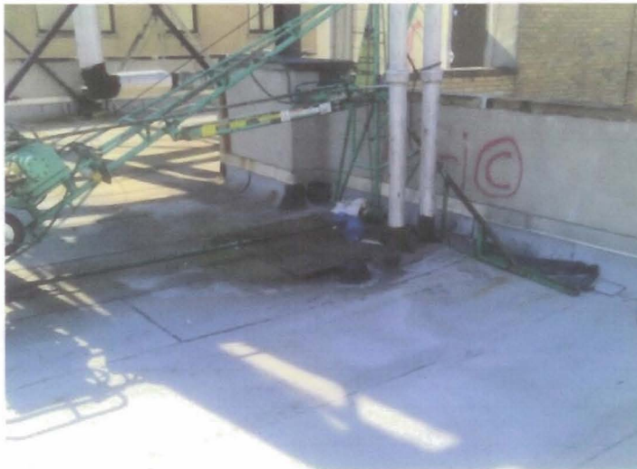
Photo 9 of 13 inadequacies 032.jpg Date: 05.10.2011 Roof - rigger hoist near parapet wall
