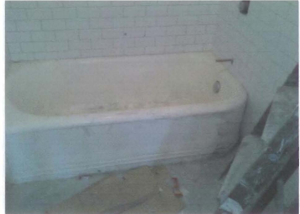
Photo 2 of 3 - Performance level – 4F bathroom
