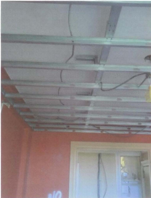
Photo 1 of 12 performance level 004.jpg Date: 05.10.2011 12F - Living Rm. electrical wiring
