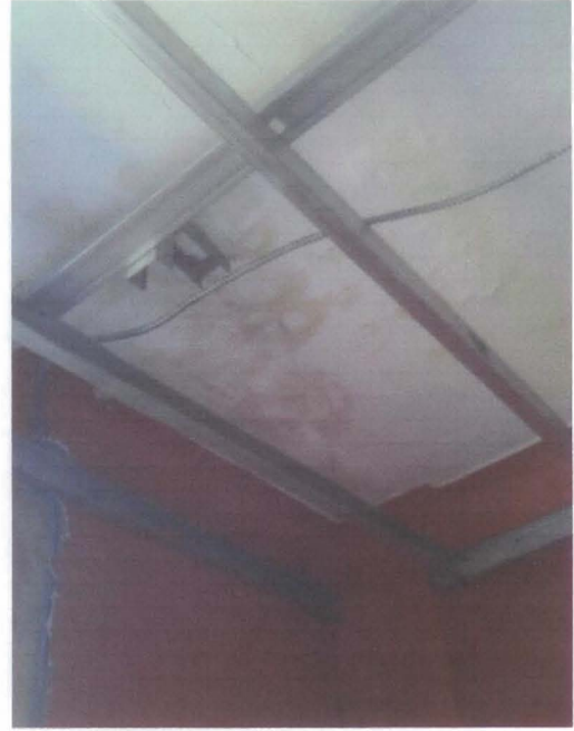
Photo 2 of 13 inadequacies 011.jpg Date: 05.10.2011 12F ceiling water damage liv. Rm.
