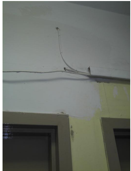
Photo 2 of 2 inadequacies Date: 11-30-2011 Loose cable wires
