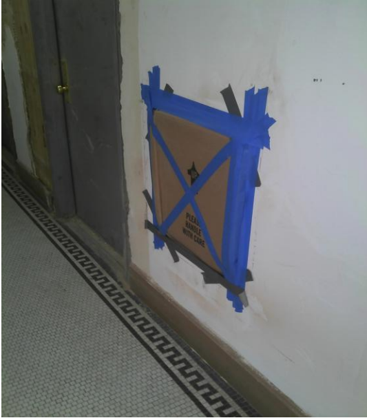
Photo 5 of 6 inadequacies Date: 11-30-2011 – Trash chute access needs Caution tape.
