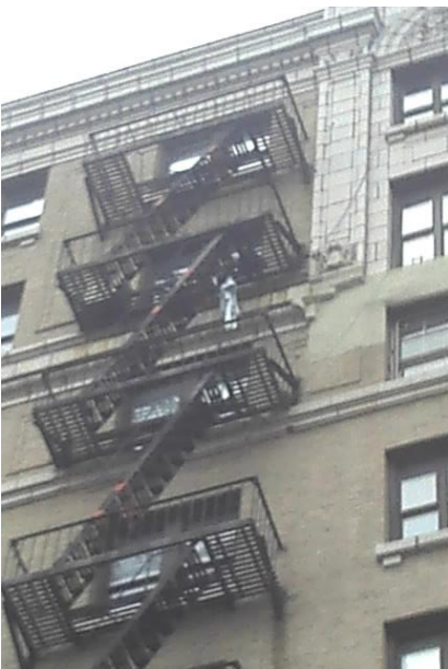
Photo 3 of 6 inadequacies Date: 11-30-2011 - Debris from fire escape
