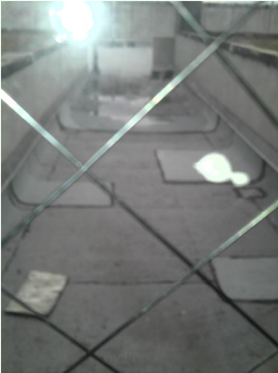
Photo 1 of 6 inadequacies Date: 11-30-2011 Roof patching
