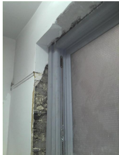
Photo 4 of 6 inadequacies Date: 11-30-2011 - New window (hall)
