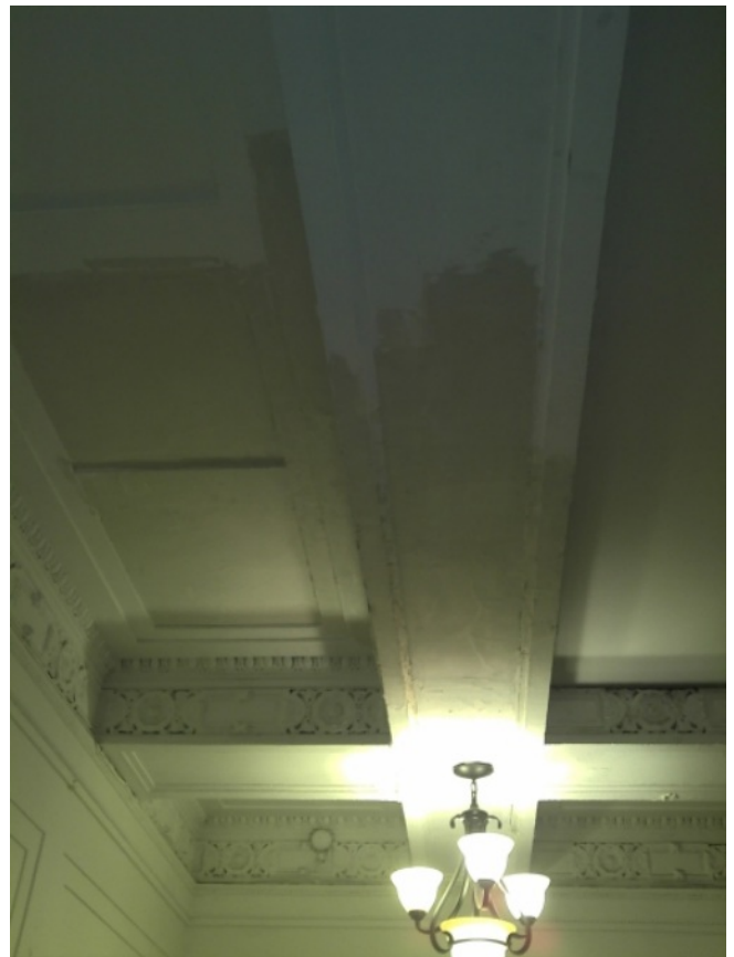
Photo 6 of 7 inadequacies 069.jpg Date: 17.11.2011 Unpained ceiling areas lobby
