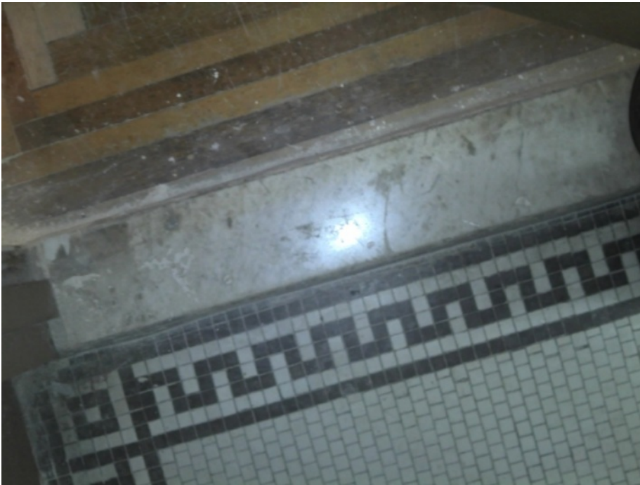
Photo 4 of 7 inadequacies 064.jpg Date: 17.11.2011 Entrance door "saddle" severe trip hazzard
