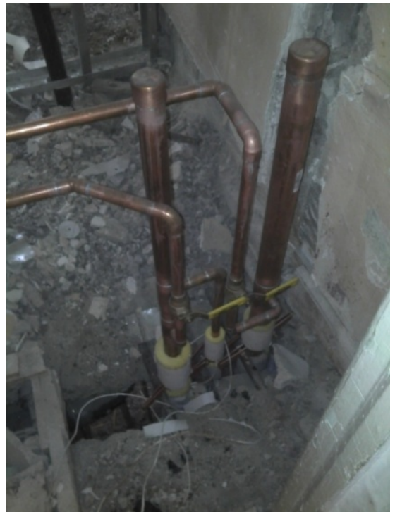
Photo 4 of 11 performance level 013.jpg Date: 17.11.2011 12F domestic water lines with cut-off valves
