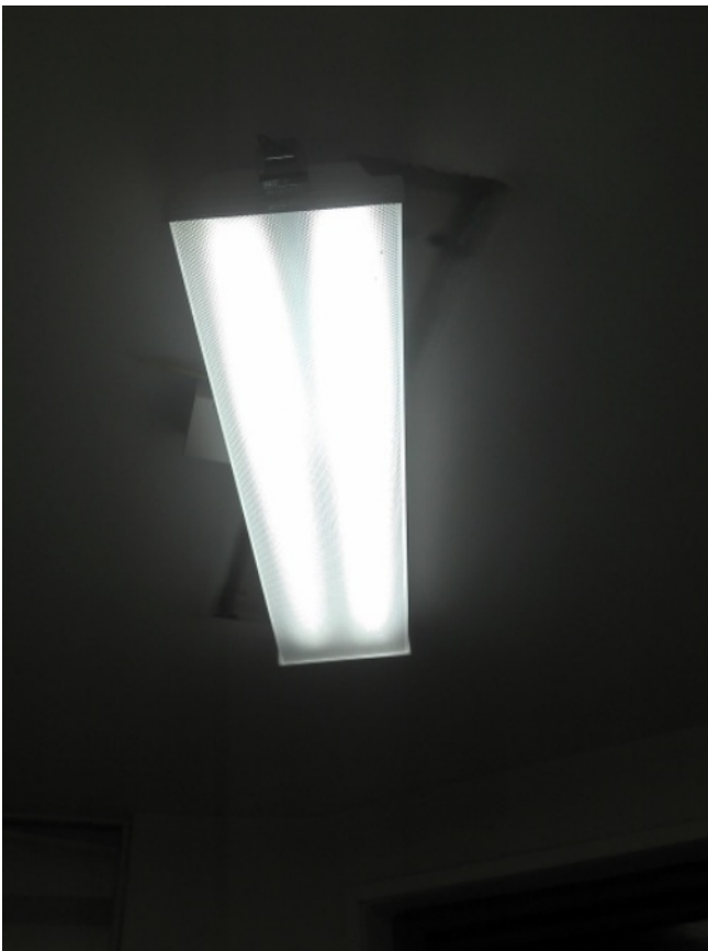
Photo 5 of 7 inadequacies 067.jpg Date: 17.11.2011 Light ajar fourth floor near elevator
