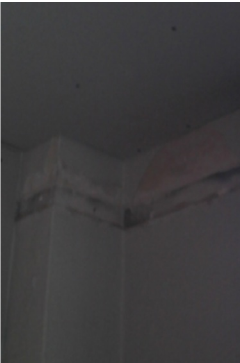
Photo 1 of 7 inadequacies 025.jpg Date: 17.11.2011 Demolished moldings 9F
