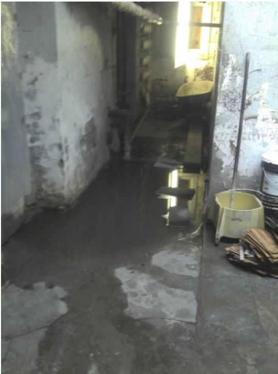
Photo 7 of 7 inadequacies 071.jpg Date: 17.11.2011 Water pooling in basement (boiler room)
