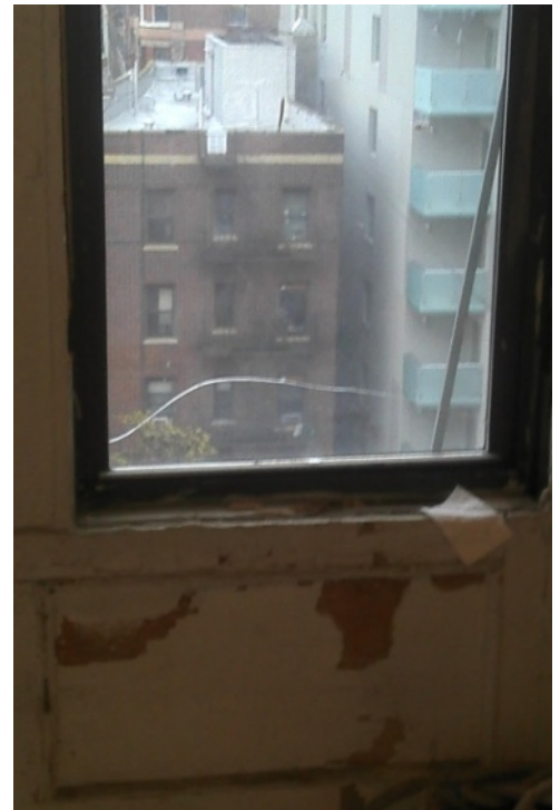
Photo 3 of 7 inadequacies 029.jpg Date: 17.11.2011 Cracked window 8F
