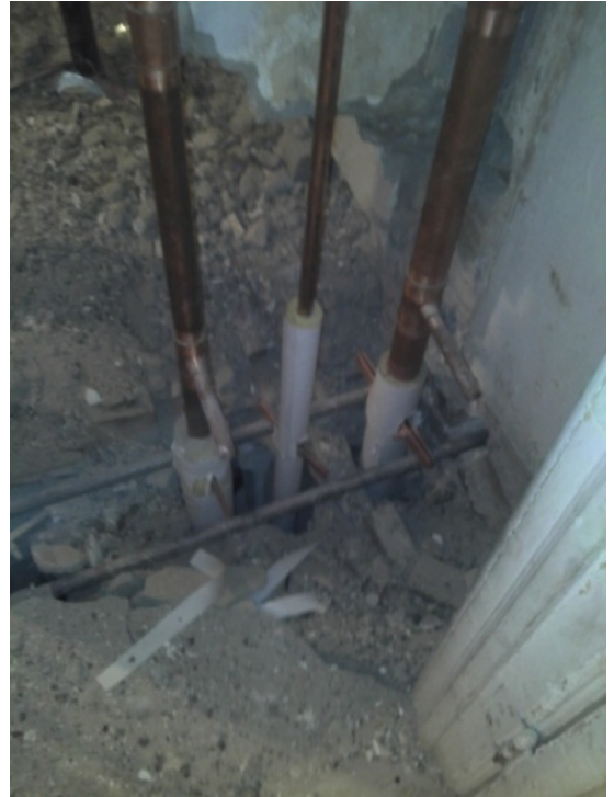
Photo 11 of 11 performance level 065.jpg Date: 17.11.2011 3F domestic water with no cut-off valves
