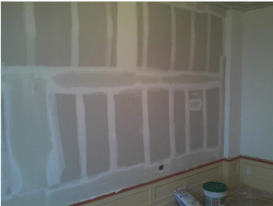
Photo 6 of 11 performance level 021.jpg Date: 17.11.2011 12F living room wall
