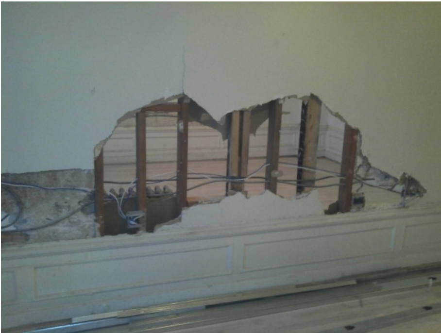
Photo 9 of 11 performance level 059.jpg Date: 17.11.2011 3F electrical wiring living room
