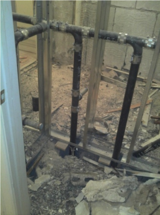
Photo 10 of 11 performance level 062.jpg Date: 17.11.2011 3F bathroom - framing and waste lines only
