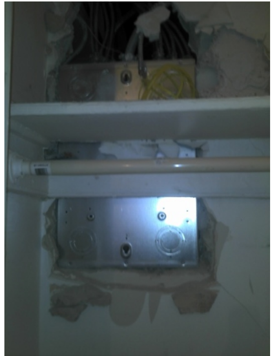
Photo 7 of 7 inadequacies 020.jpg Date: 17.11.2011 12F Hall closet electric box back
