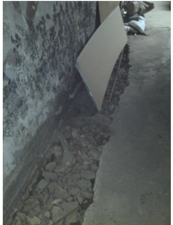
Photo 3 of 3 inadequacies 097.jpg Date: 17.10.2011 Basement - floor trenching
