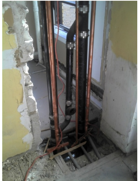
Photo 2 of 9 performance level 007.jpg Date: 17.10.2011 11F Kitchen waste, water and gas piping
