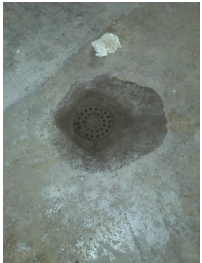
Photo 1 of 3 inadequacies 107.jpg Date: 17.10.2011 Laundry Room (basement) floor drain
