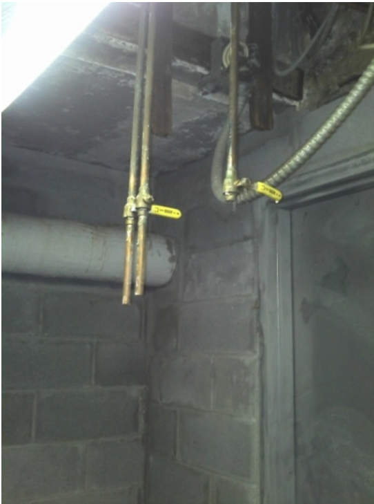
Photo 2 of 3 inadequacies 095.jpg Date: 17.10.2011 Basement - water line leaking
