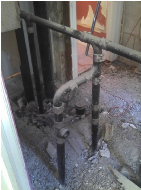
Photo 3 of 9 performance level 009.jpg Date: 17.10.2011 11F Bathroom piping
