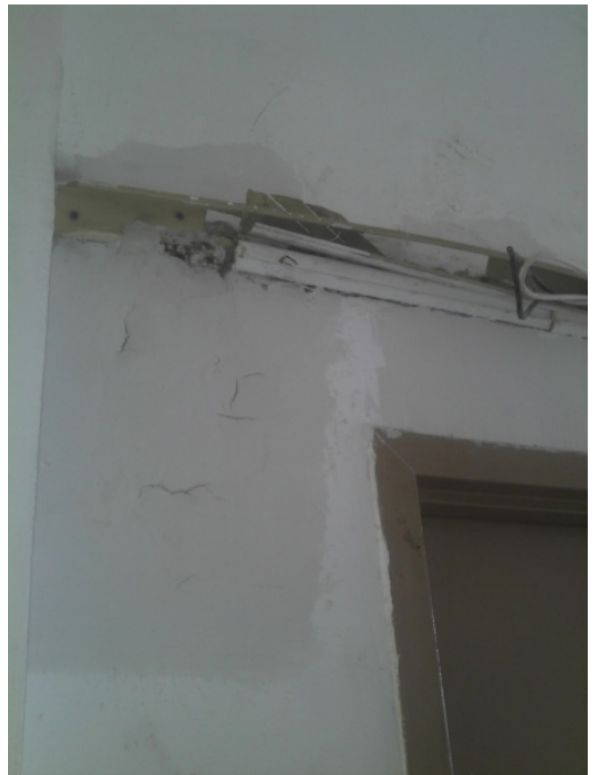
Photo 13 of 13 inadequacies 019.jpg Date: 05.10.2011 12th floor hallway - poorly finished wall "prep" and paint
