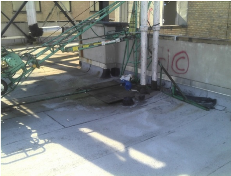
Photo 9 of 13 inadequacies 032.jpg Date: 05.10.2011 Roof - rigger hoist near parapet wall
