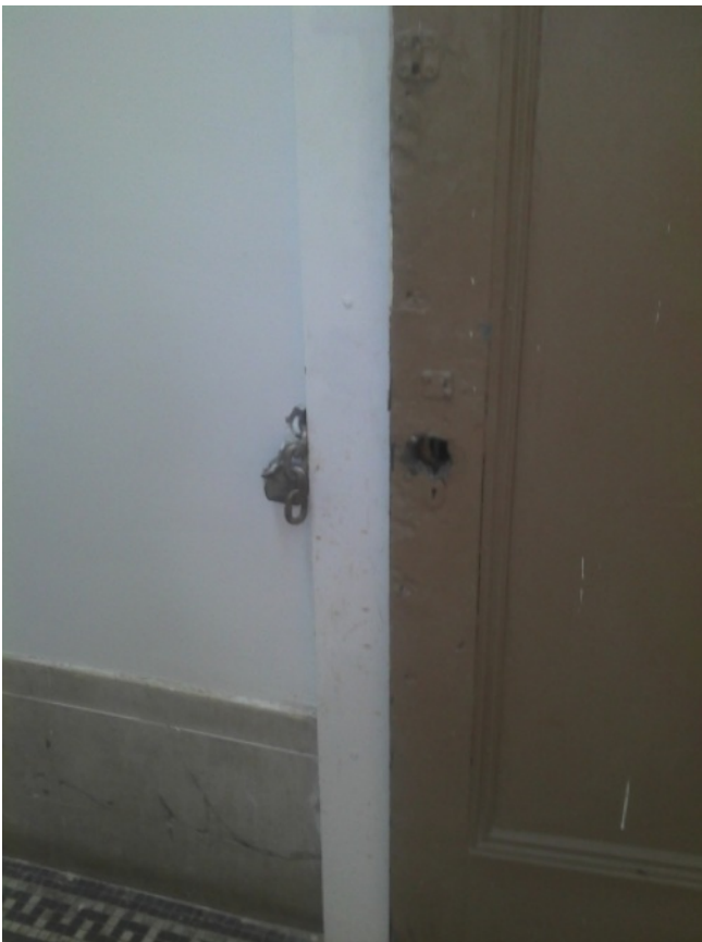
Photo 12 of 13 inadequacies 042.jpg Date: 05.10.2011 Mail room - storage room door hardware missing
