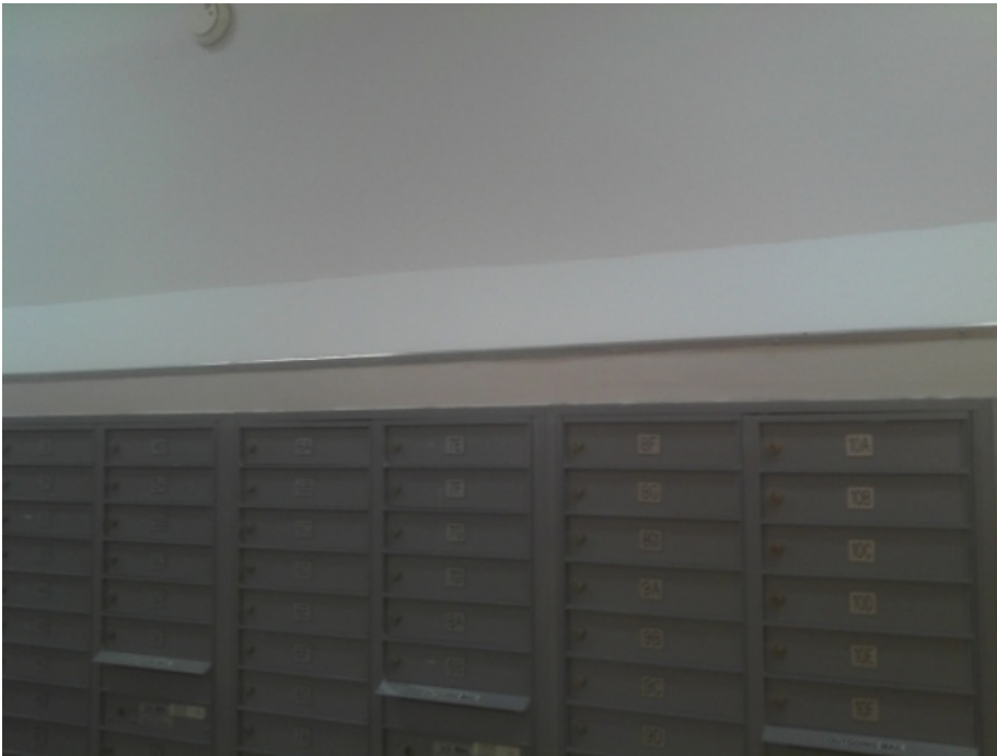
Photo 11 of 13 inadequacies 041.jpg Date: 05.10.2011 Mail room - finish
