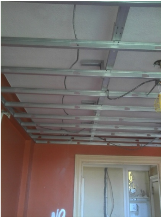
Photo 1 of 12 performance level 004.jpg Date: 05.10.2011 12F - Living Rm. electrical wiring
