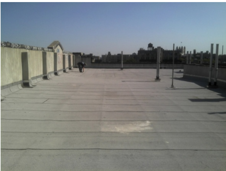
Photo 7 of 13 inadequacies 025.jpg Date: 05.10.2011 Roof
