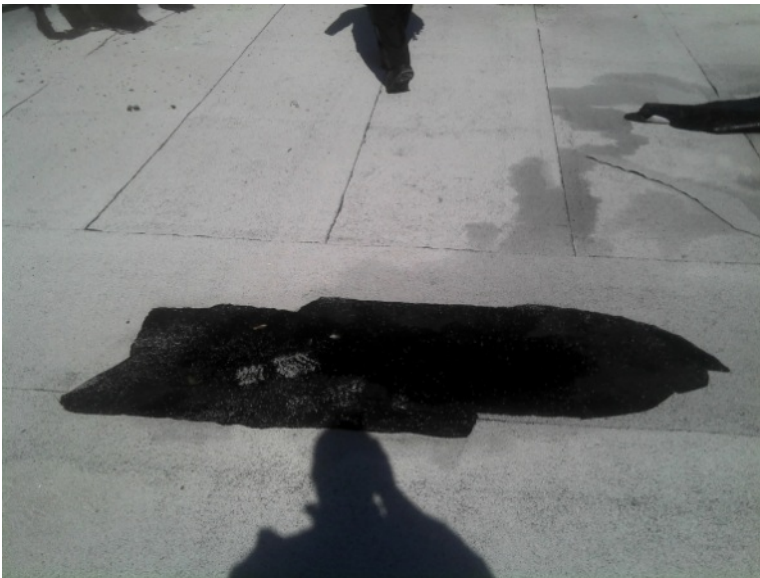
Photo 6 of 13 inadequacies 024.jpg Date: 05.10.2011 Roof - damage to external membrane
