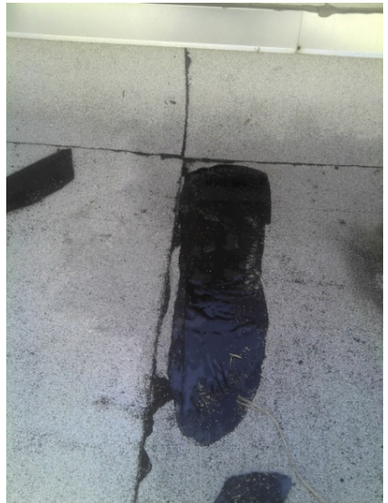
Photo 4 of 13 inadequacies 022.jpg Date: 05.10.2011 Roof - damage to external membrane
