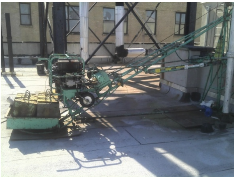
Photo 10 of 13 inadequacies 033.jpg Date: 05.10.2011 Roof - rigger hoist near parapet wall
