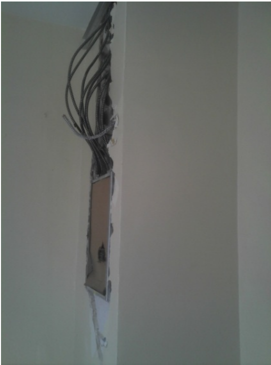
Photo 5 of 12 performance level 013.jpg Date: 05.10.2011 12F Kitchen electric box
