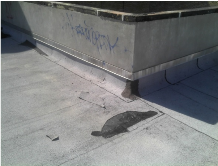
Photo 8 of 13 inadequacies 029.jpg Date: 05.10.2011 Roof - damage to external membrane near parapet wall
