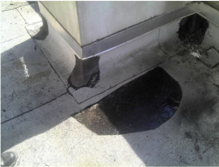
Photo 5 of 13 inadequacies 021.jpg Date: 05.10.2011 Roof - damage to external membrane
