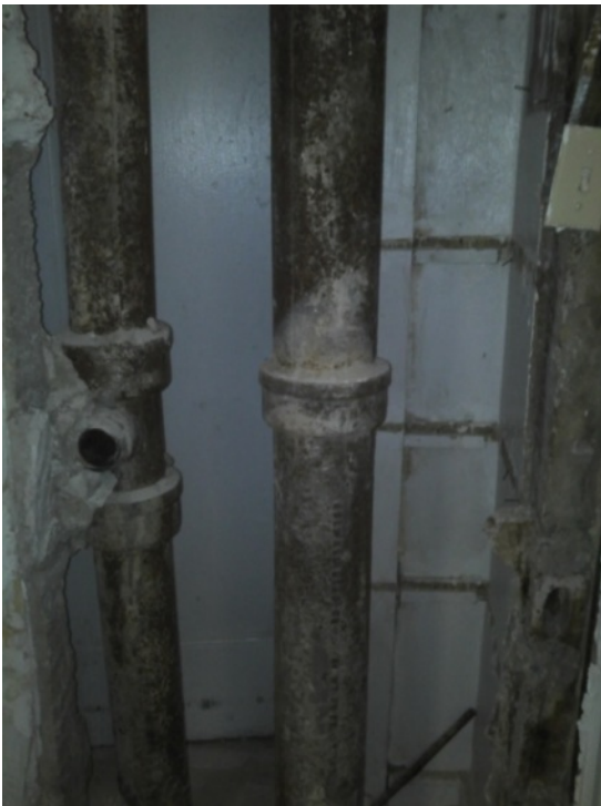
Photo 2 of 3 inadequacies 037.jpg Date: 14.09.2011 Galvanized Pipe bathroom 10F
