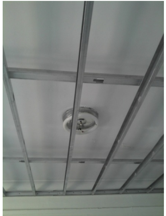
Photo 1 of 3 inadequacies 042.jpg Date: 14.09.2011 Ceiling frame 8F bedroom
