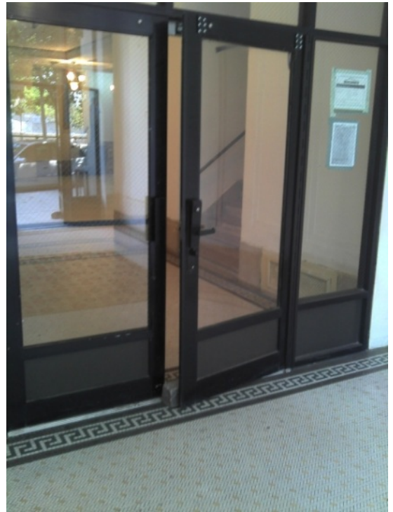
Photo 3 of 4 inadequacies 012.jpg Date: 13.09.2011 Vestibule door ajar
