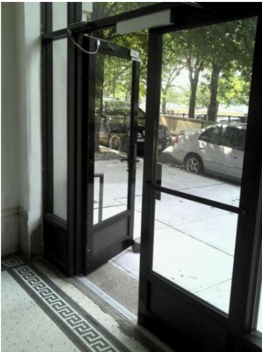
Photo 4 of 4 inadequacies 010.jpg Date: 13.09.2011 Entrance door ajar
