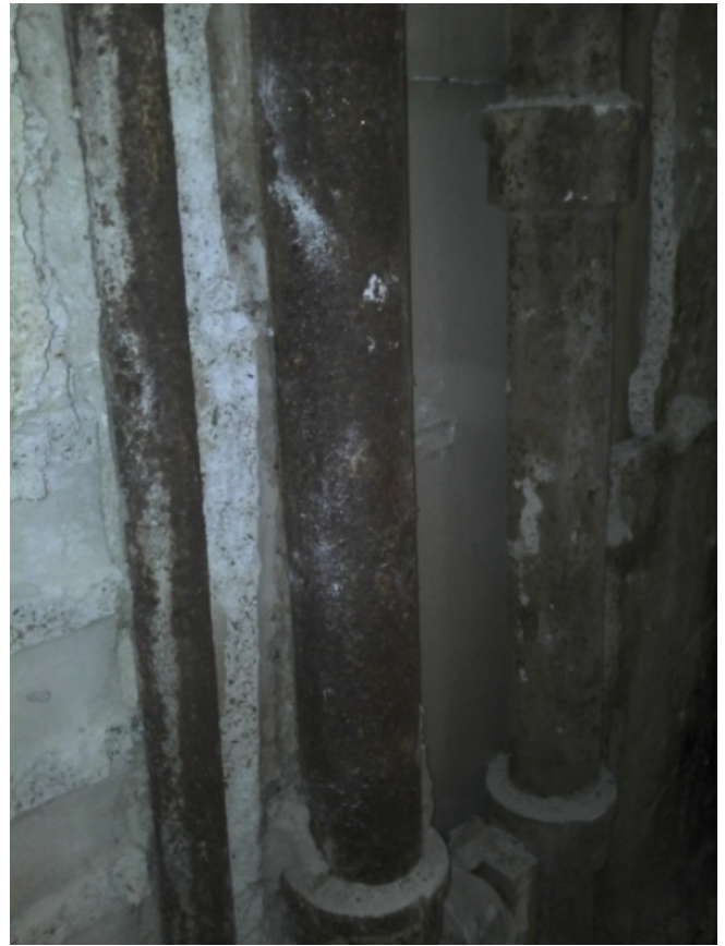
Photo 2 of 4 performance level 022.jpg Date: 13.09.2011 Waste and water lines
