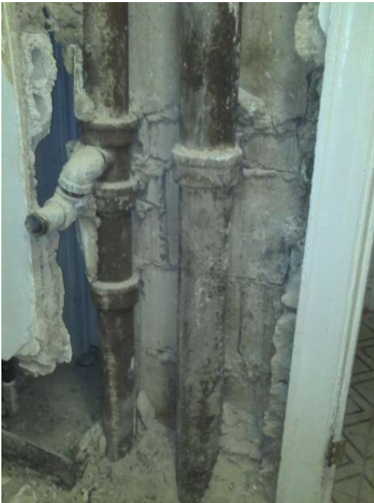
Photo 2 of 4 inadequacies 015.jpg Date: 13.09.2011 Galvanized piping bathroom 7F (waste line)
