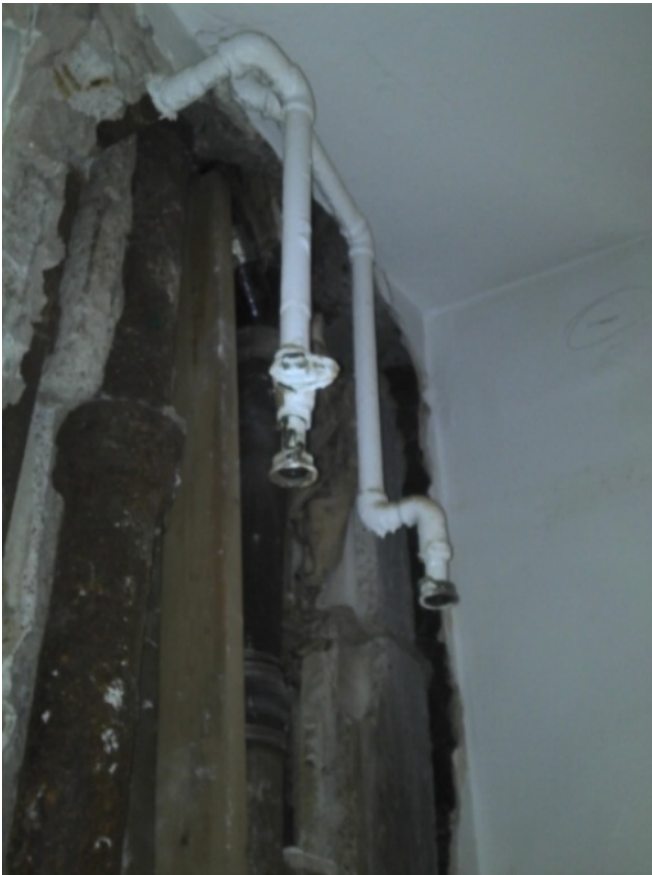
Photo 4 of 4 performance level 026.jpg Date: 13.09.2011 Waste water and gas lines kitchen 7F
