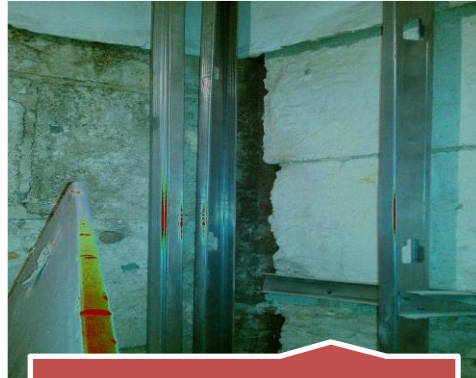
Inadequacies: G1 rear bathroom, wall furring and imbedded existing waste riser affecting E line.
