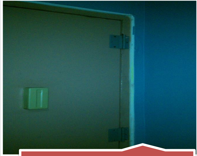
Inadequacies: Incorrect door hinges in apartment 5A
