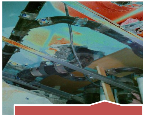
Inadequacies: Tight network of waste line pipes.
