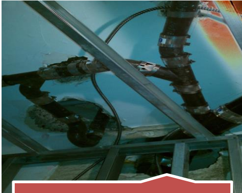
Performance level: Exposed waste lines.
