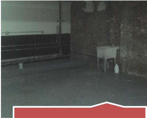
Inadequacies: Laundry room inadequate lighting.
