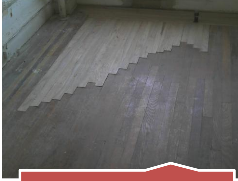
Inadequacies: Wood floor trip hazard
