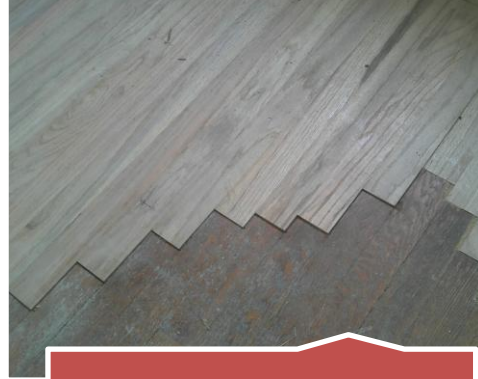
Inadequacies: Wood floor trip hazard
