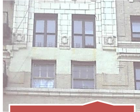
Inadequacies: 10th floor wood frame window
