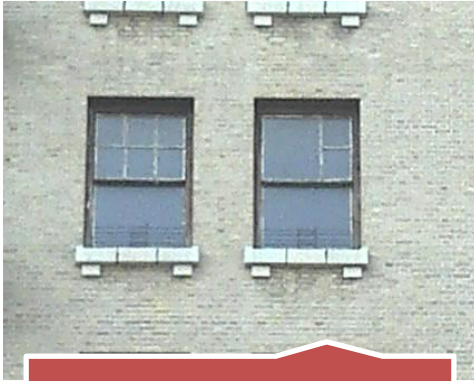
Inadequacies: 6th floor wood frame window
