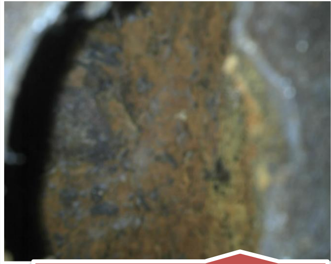
Inadequacies: Inside cut galvanized
