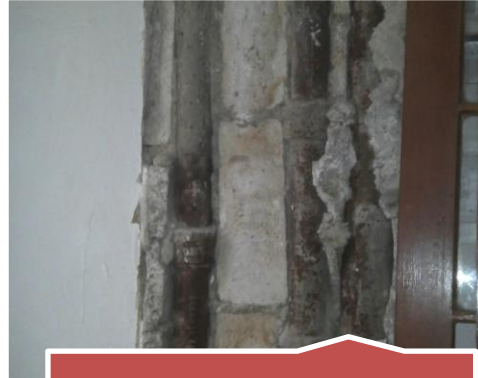
Inadequacies: 12G exposed waste line.
