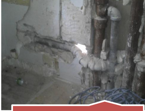
Inadequacies: Exposed waste line unit 12G bathroom..
