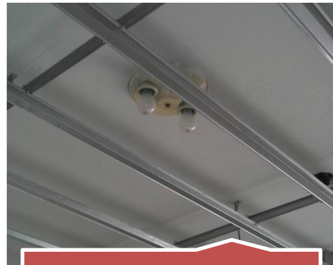
Inadequacies: Framing for ceiling drop (11G).
