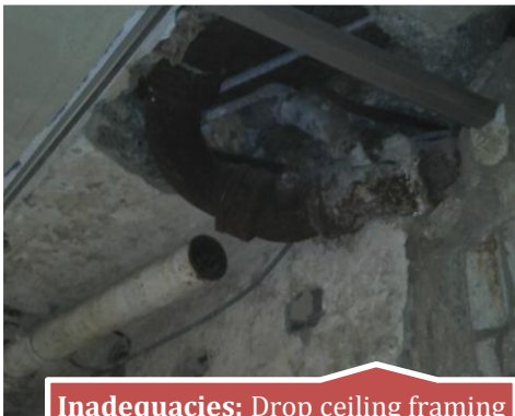
Inadequacies: Drop ceiling framing with exposed waste line and old disconnected line which needs to be removed (7G).
