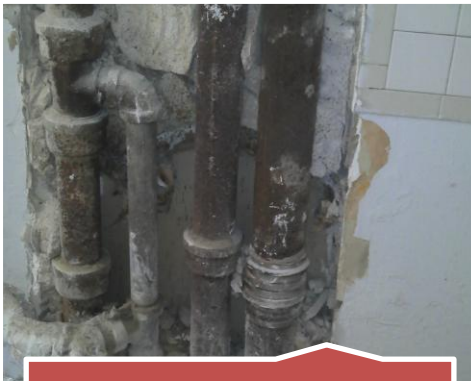
Inadequacies: Exposed galvanized waste lines 11G
