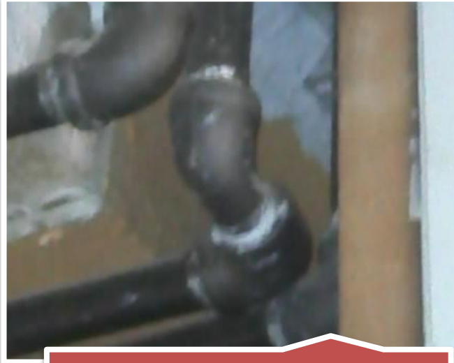
Inadequacies: Incorrectly installed double elbow for gase line.
