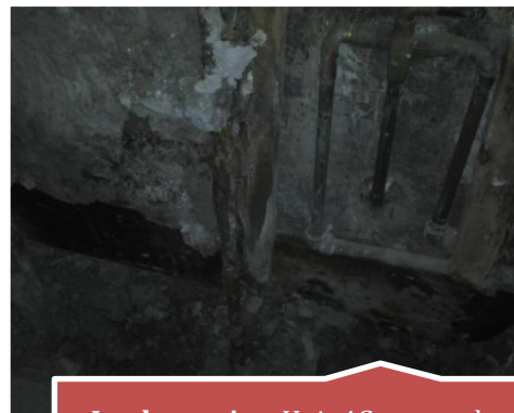
Inadequacies: Unit 4G exposed waste line, shared with E line. Exposed bathroom plumbing E line.
