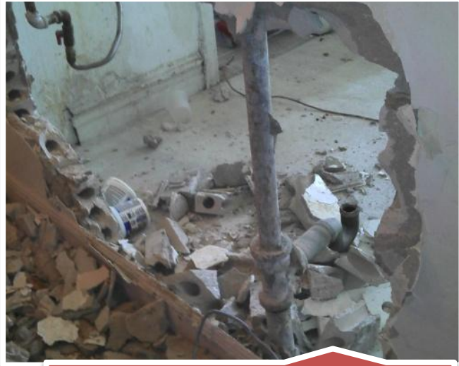
Inadequacies: Unit G41, kitchen waste pipe. Smaller than code requirement.
