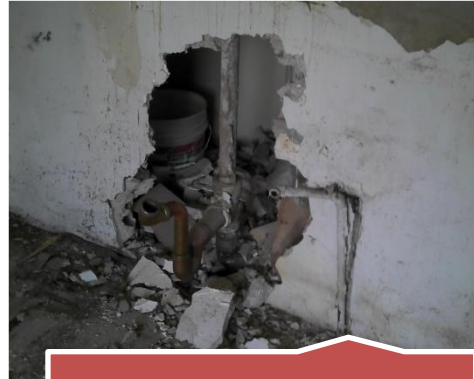
Inadequacies: Kitchen waste line. Smaller than what is required by code. this line should be replaced
