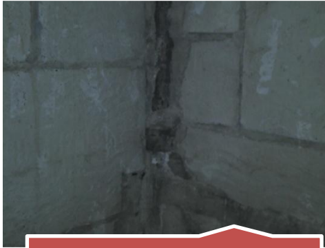
Inadequacies: Exposed waste line unit 7G bathroom. Shared line with E line unit.
