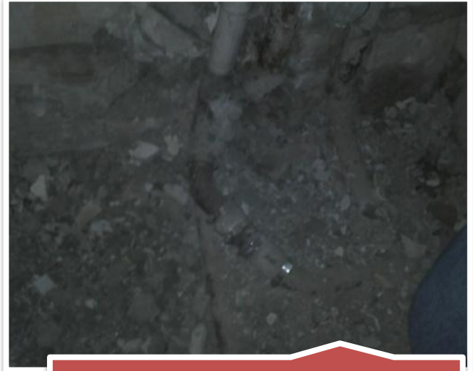
Inadequacies: Waste line tie.
