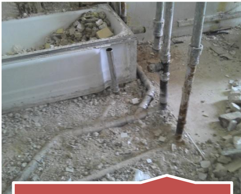
Inadequacies: Severely limited capacity waste line from kitchen
