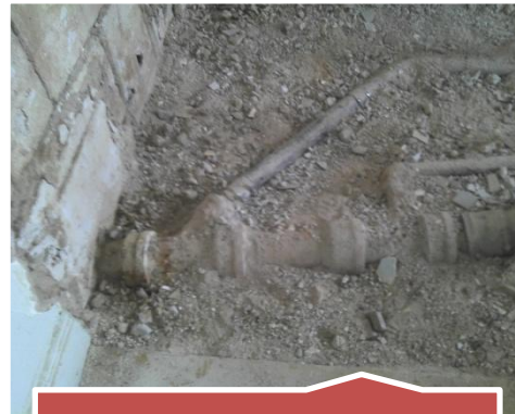
Inadequacies: Waste line ties to main line.
